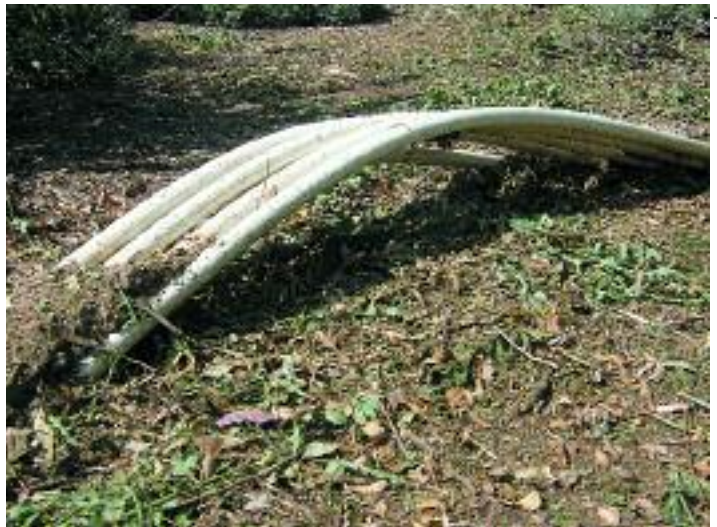
Irrigation pipes arching out of the ground, as a result of the shifting and settling soils at the South Coast Botanic Garden
