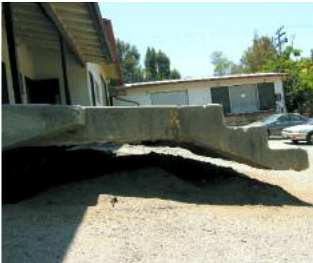
The steps to the original administration complex after settling of the soil due to continual decomposition of buried trash in the former landfill site
